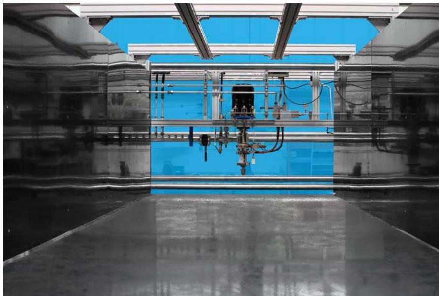
Hennecke's new slabstock plant: continuous foam production with extremely compact dimensions
